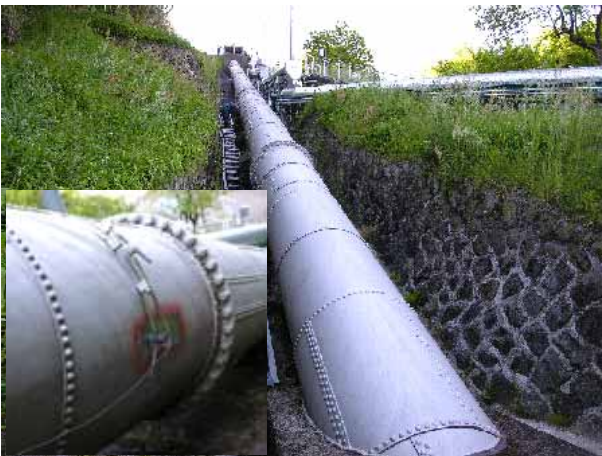
Figure 10 Overview of measurement test at a steel penstock in a hydro-power station.
