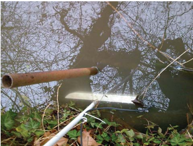
Figure 2: UB-Flow F156 installed on the river Aar.
